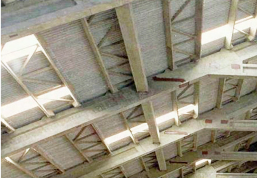
Fig 7.4: Slab units on trussed purlins, supported on rafters of A-frames (Silo at Thoothukudi)
