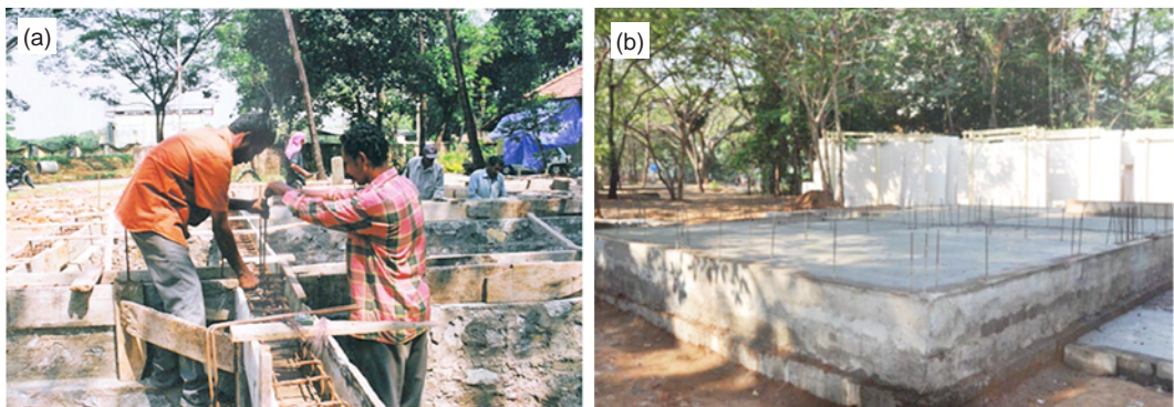
Fig. 4.8: (a) Insertion of rebars, and (b) foundation with starter bars in position
