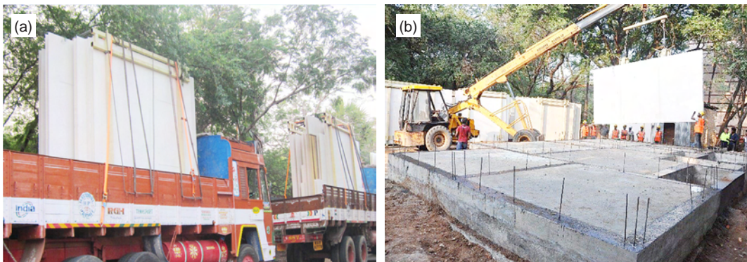
Fig. 4.9: (a) Arrival of wall panels to site in trucks, and (b) wall panel being lifted using crane
