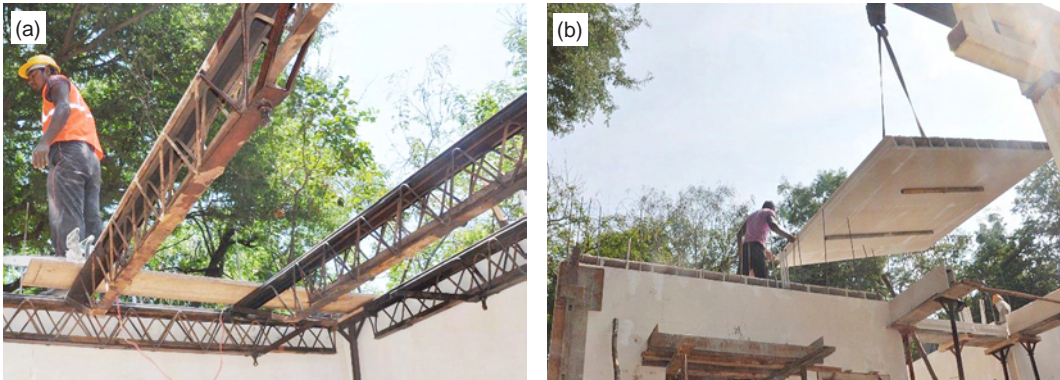
Fig. 4.13: (a) Propping done for the placement of GFRG slab, and (b) panel lifted using two spreader bars
