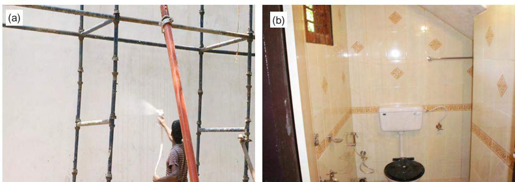
Fig. 4.17: (a) Spraying of primer on GFRG panel surface, and (b) glazed tiles fixed over the GFRG panel surface using special adhesive
